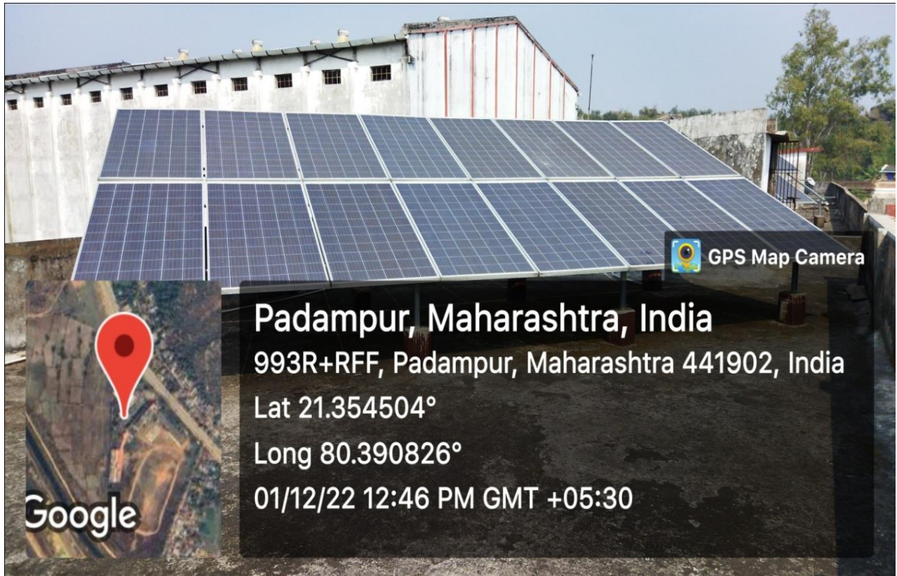
Photoelectric Power Generation – Unit 1
