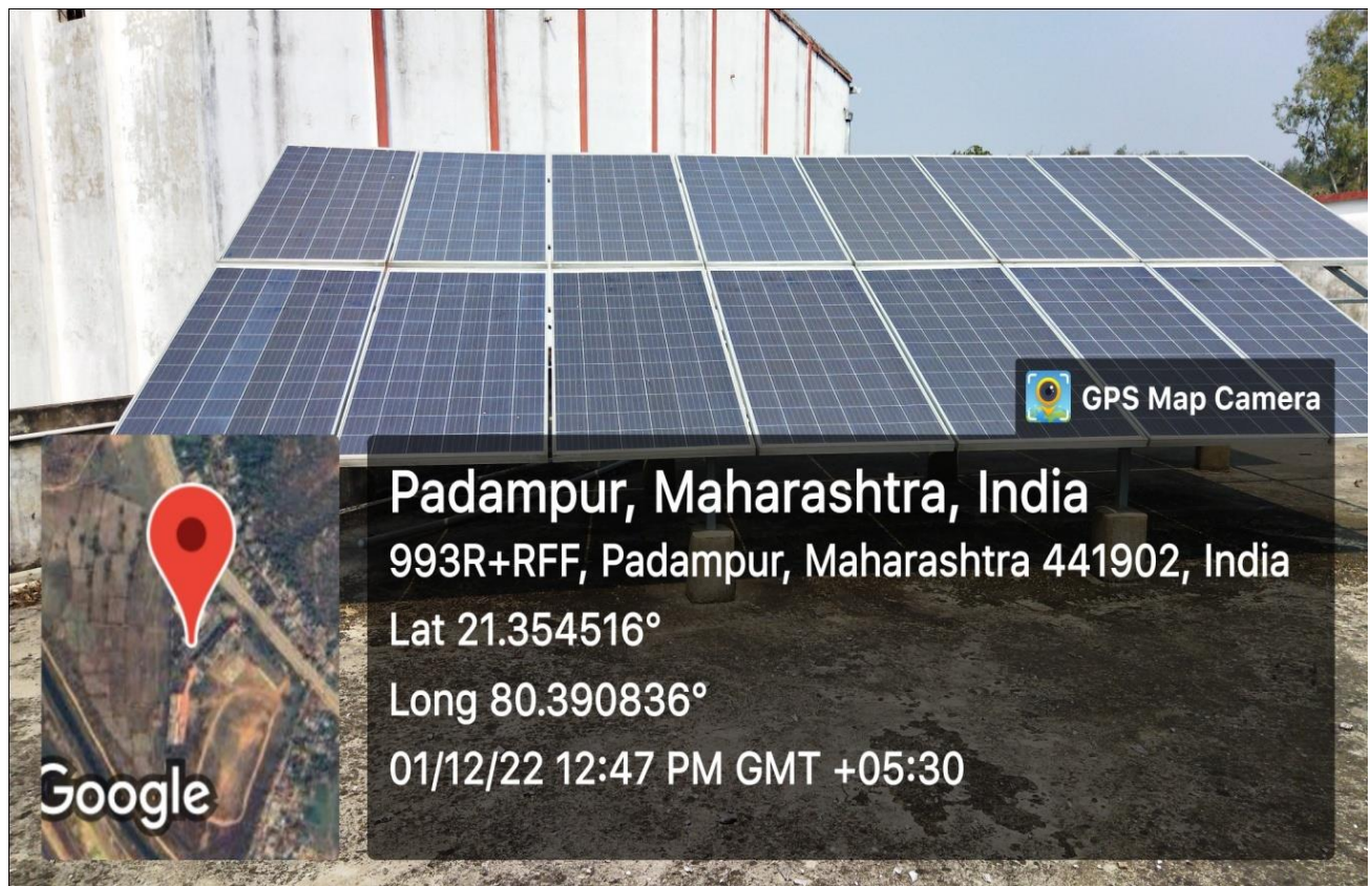
Photoelectric Power Generation – Unit 2
