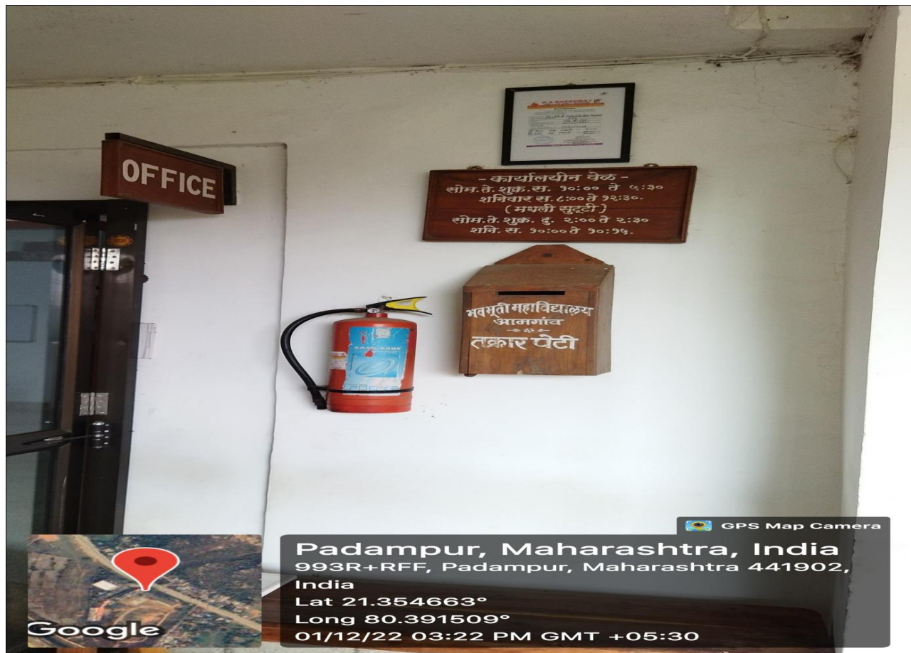
Complaint Box/Fire Extinguisher
