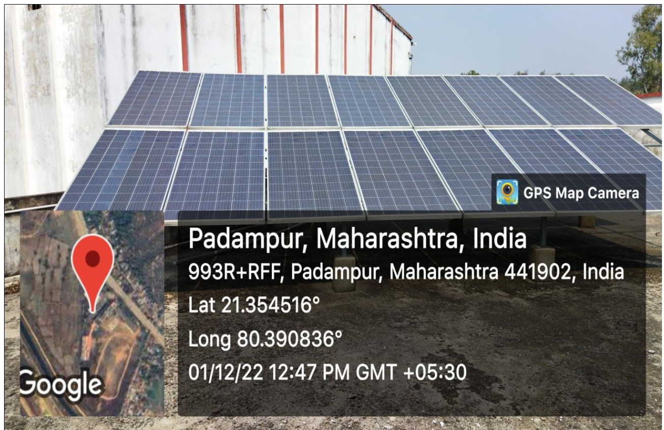
Photoelectric Power Generation – Unit 2
