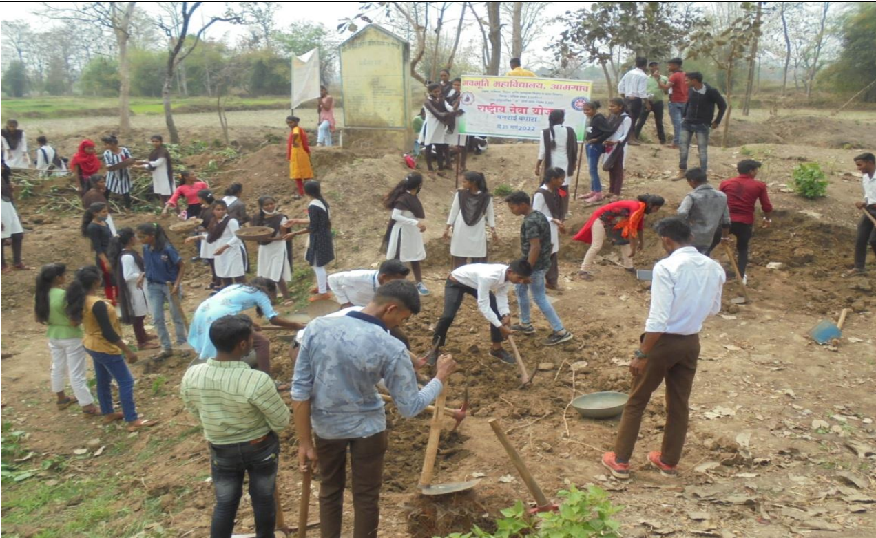
Labor activity of NSS students to built a clay barrier at village canal at the village Jamkhari, Tahsil Amgaon, during NSS special camp
